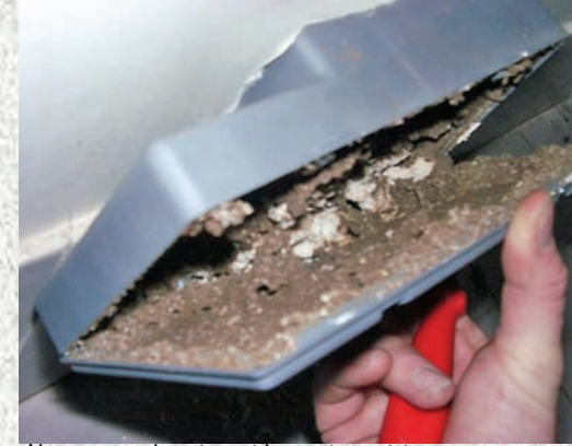
Above ground station with termite activity.
