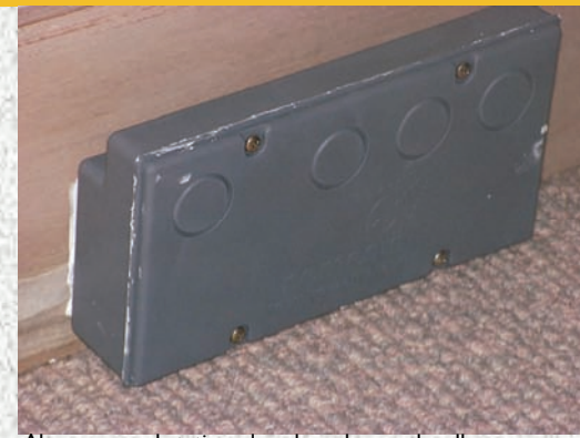
Above ground station placed on damaged wall.
